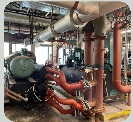
Aged and Inefficient Equipment and Materials
