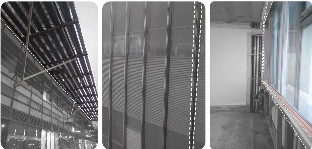
Figure 3.24 Images of aluminium components in the building. Wind canopy (left), facade mullion (middle) secondary frame (right)
