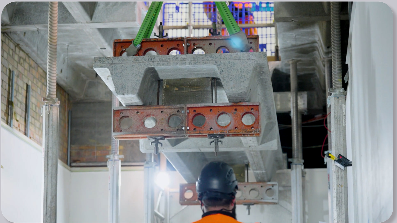
Figure 2.19 Image showing the slab specimen being lowered for removal to the ground floor
