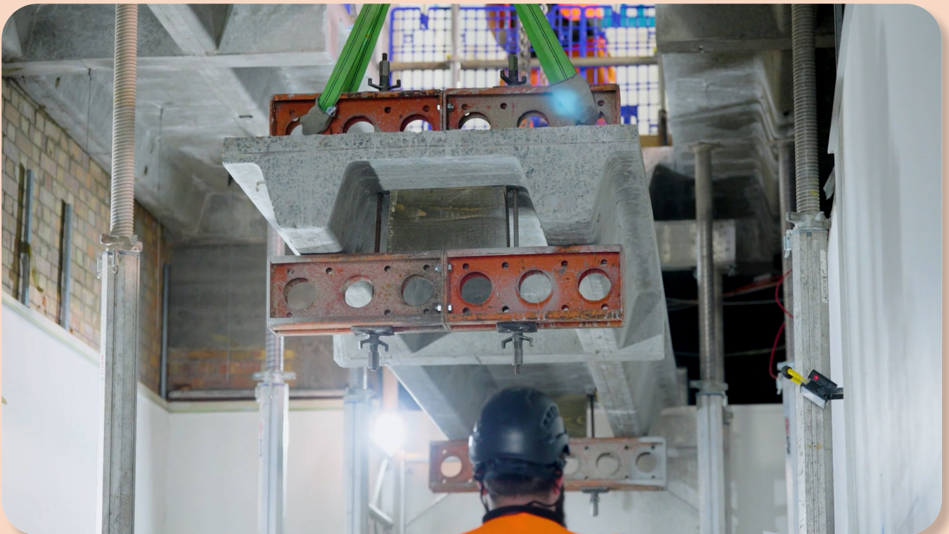
Figure 3.11 Image showing the slab specimen being lowered for removal in the ground floor corridor.
