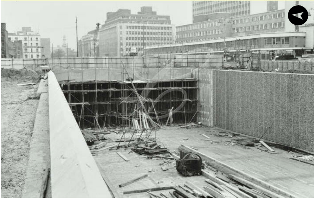
Figure 8 - Euston Road Underpass under construction ~1966 Source- A London Inheritance/ London Metropolitan Archives https://alondoninheritance.com/london-streets/a-lost-bank-and-the-adam-and-eve-pub-on-the-corner-of-euston-road-and-hampstead-road/attachment/eus
