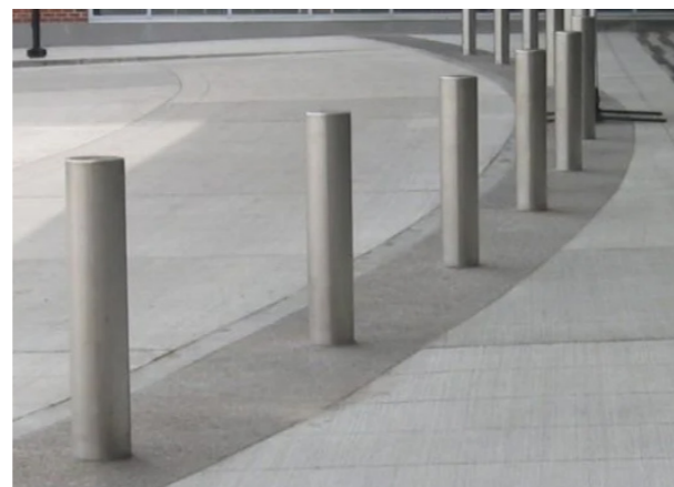
O1 When there is the absence of a mound, the security line is supported by bollards
