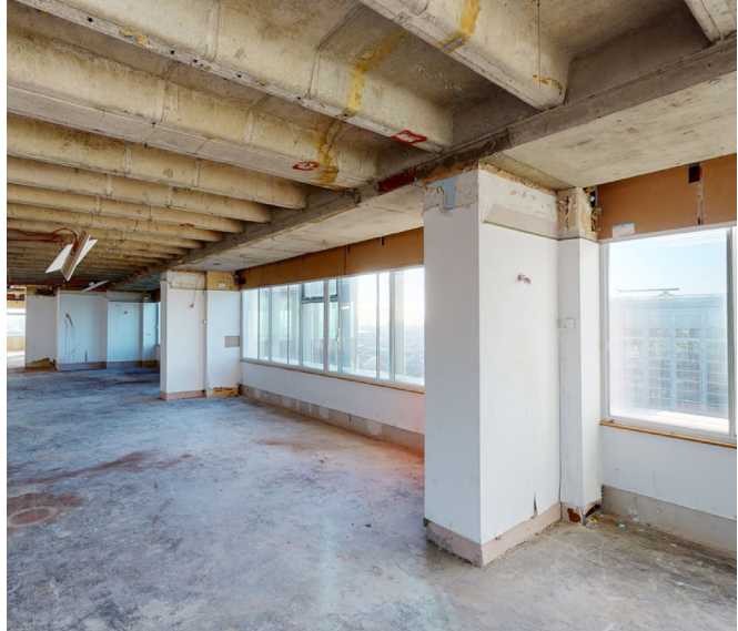
Figure 16.11 Existing ring beam is deeper than the rest of the structural floor system, creating a pinch point for clear floor to ceiling heights once new ceiling services are installed
