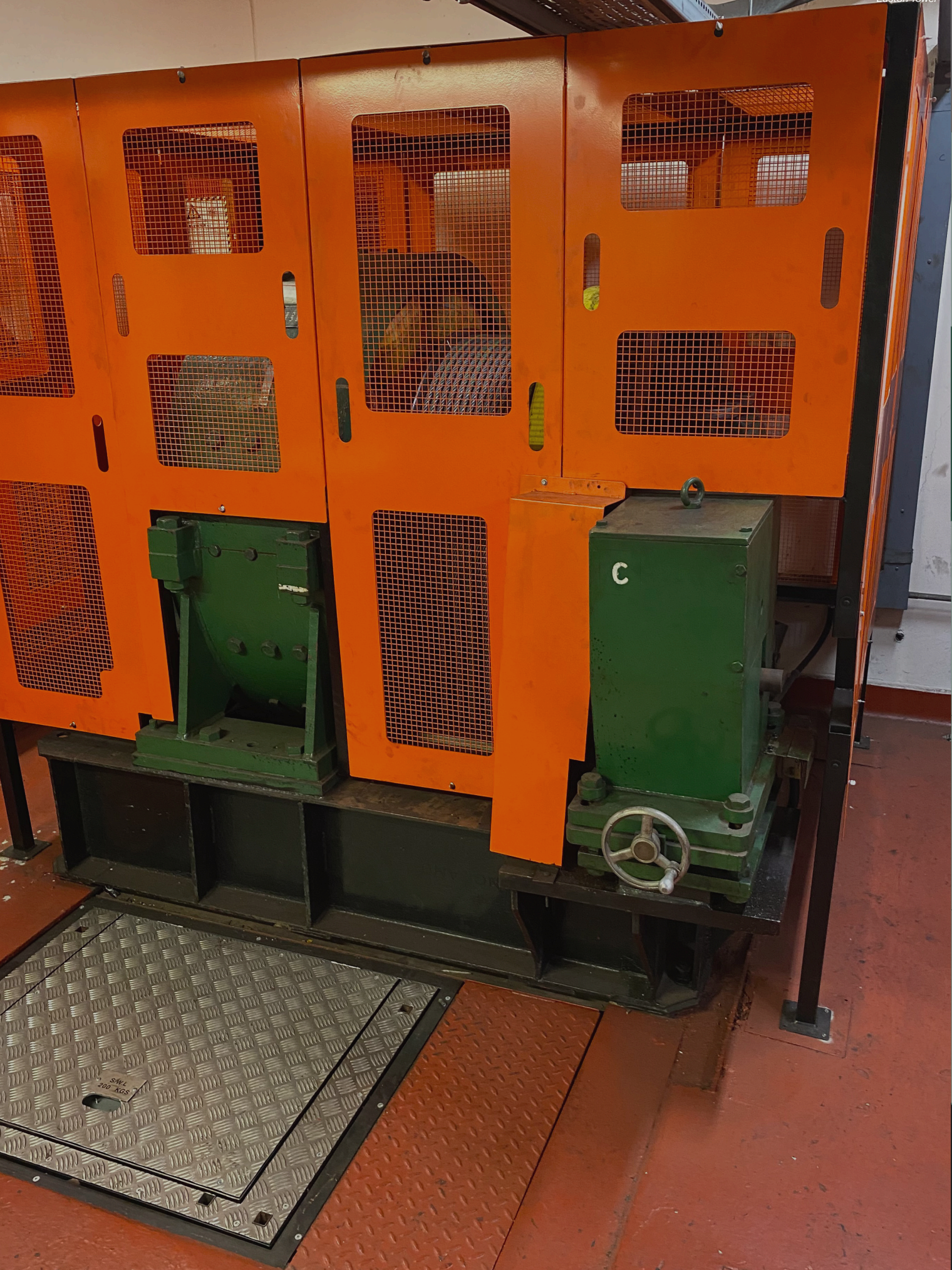
Figure 9.21 Existing high rise lift motor at Euston Tower
